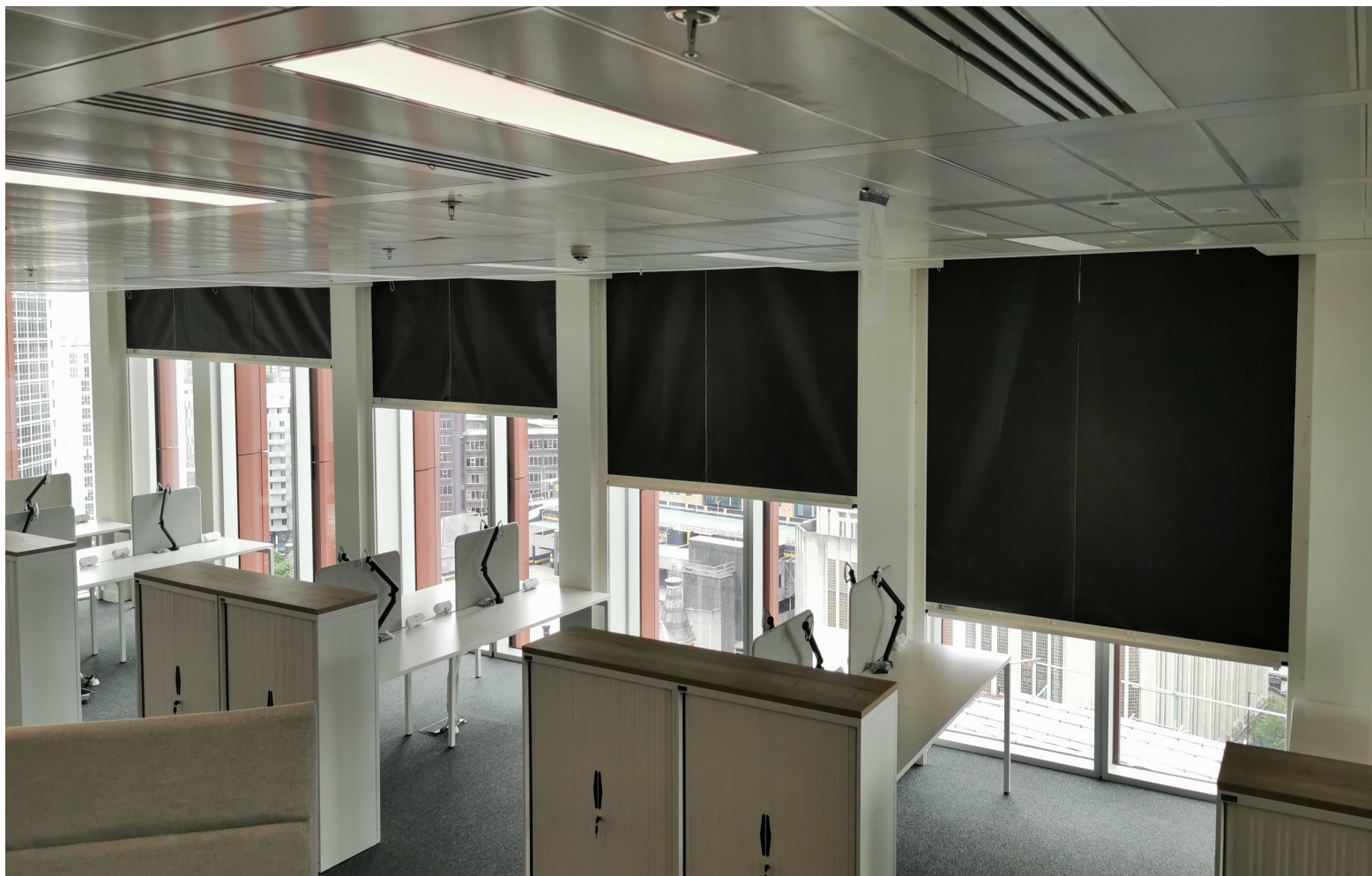
Flameshield EW 120 Fire Curtains installed in Manchester s Deansgate
